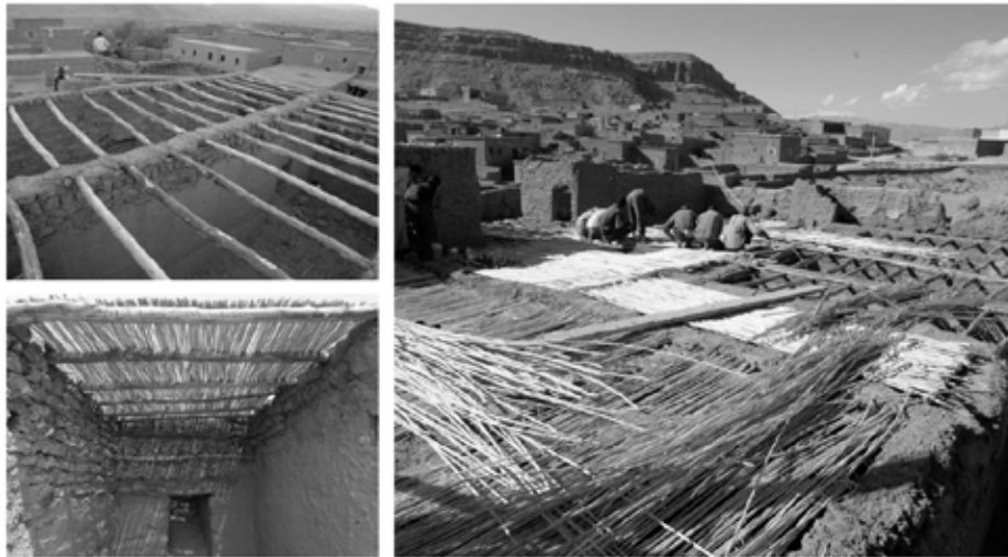
Fig. 2.31 Colocación techo de cañizo. Boussalh, M. (2005). Conservation manual for earth architecture heritage in the pre-Saharan valleys of Morocco . Ministry of Culture.
